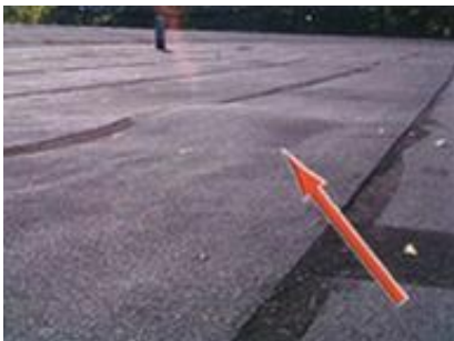
BLISTER UNDER ROOF MEMBRANE
