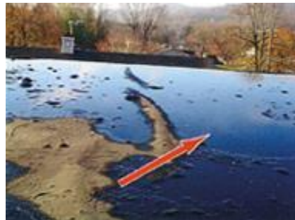
EXCESSIVE WEIGHT DUE TO PONDING
